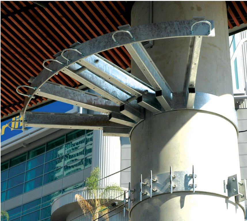
Custom steel column brackets used for the specialized suspended lighting system at the 2008 Luminato® Festival in Toronto
