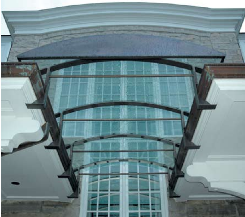
Designed to drain into existing eaves troughs
