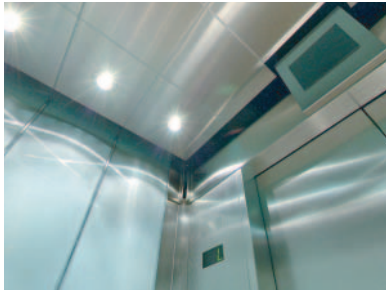
Brushed st. stl. ceiling with recessed pot lights and 'Captive Network' ready monitor
