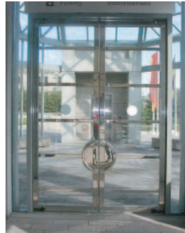
A set of st. stl. entrance doors, exterior
